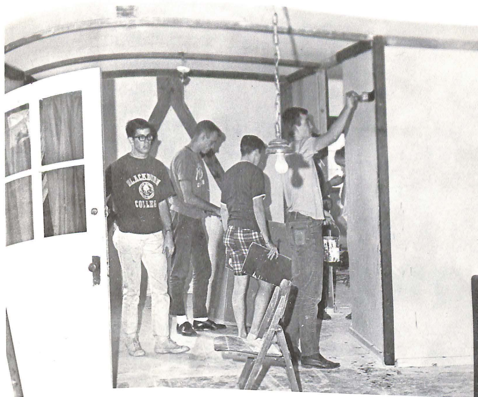
ABOVE: The work crew add the finishing touches to the Bell, Book, & Candle after a long, hard work session.
